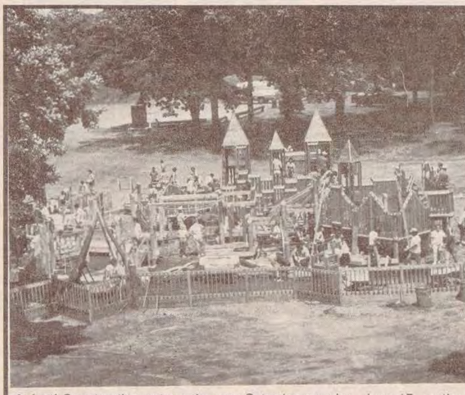
At last! Construction gets under way Saturday morning, June 15, on the Maplewood Community Playground-- More pictures - page 13.
