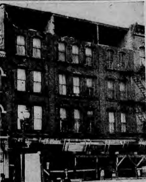
AWAITING REPAIRS — Six weeks after it partially collapsed, the building at 114-120 Main St. W. still awaits repairs.
