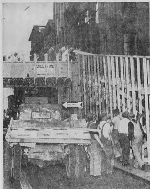
Half a hundred or more carpenters swing ramp frame into position. Lumber for structure was box lumber which will be salvaged and returned to regular uses as soon as bridge comes down.
