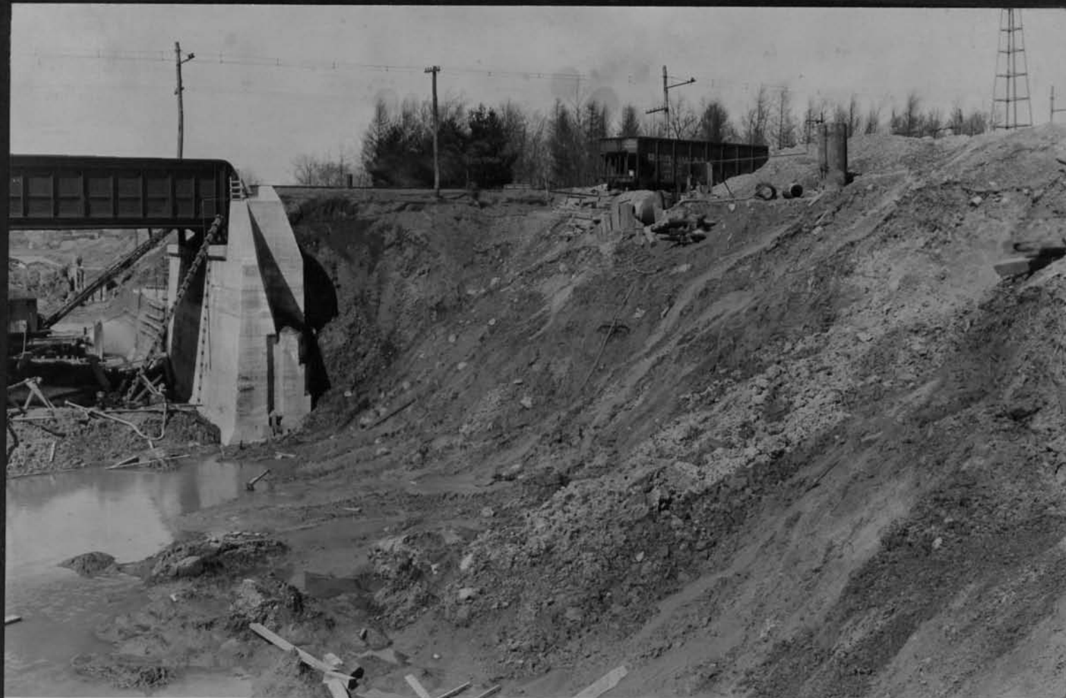
11679 Slide in north bank at L V R R crossing Looking west Cont 59 March 22 1918
