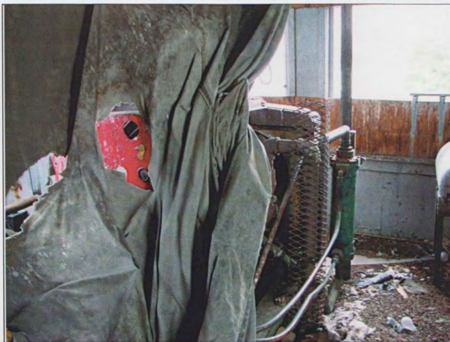
Figure 14. Machine room in the control house.
