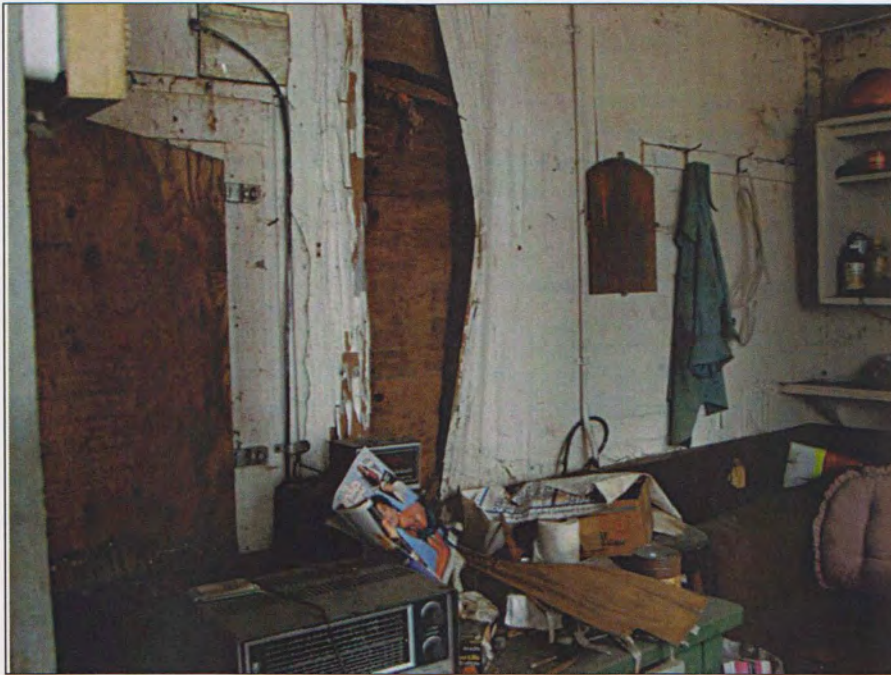
Figure 11. Interior office area of control house.
