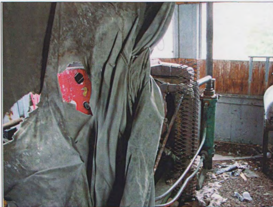
Figure 14. Machine room in the control house.
