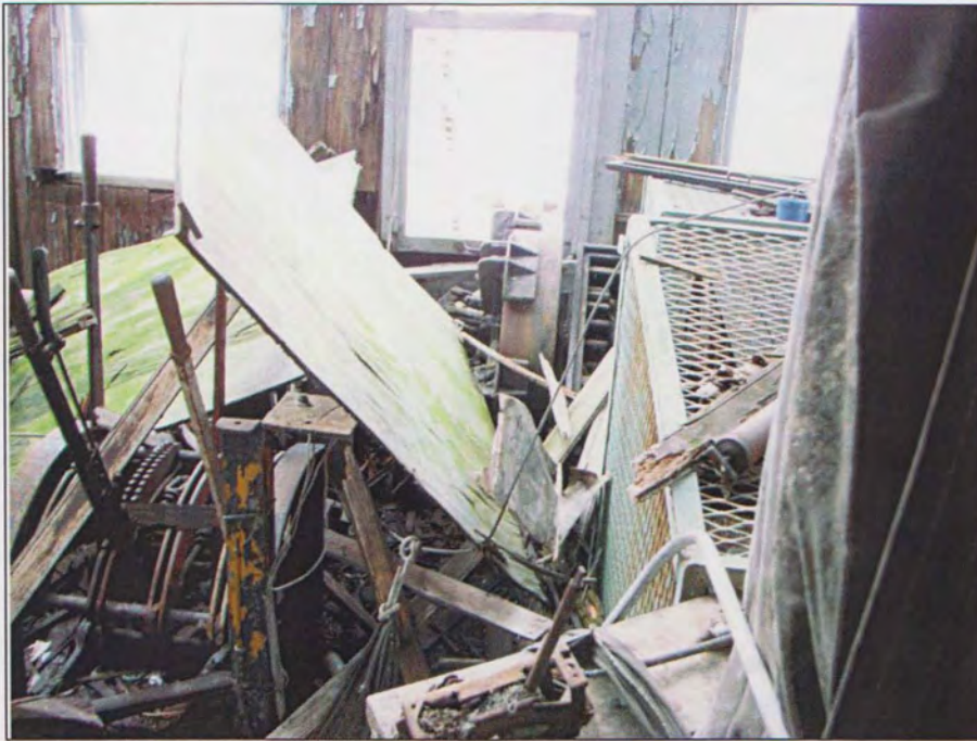
Figure 13. Machine room in the control house.
