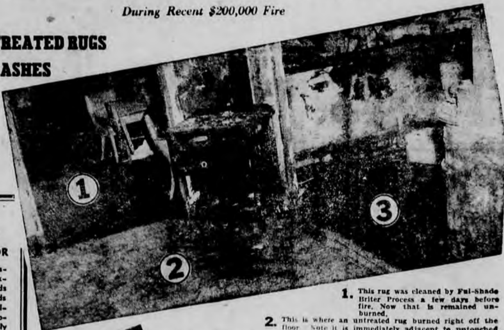
Actual Photo of Interior After Fire
